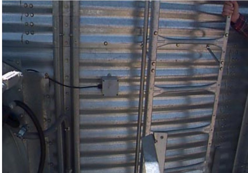
Plenum temperature sensor on the bin sidewall.
